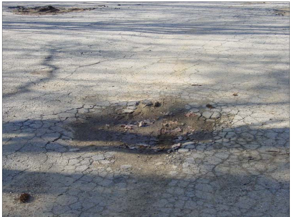
Welcome to the H.S.A - When you come through the gate into the parking lot this pot hole is there to greet you. A few years ago this hole was not there. Now it has grown to 3 feet in diameter and 6 inches in depth. Note the broken asphalt around the pot hole. In the upper left hand corner of the photo is a new area that has just failed this winter and is now starting to break up.
