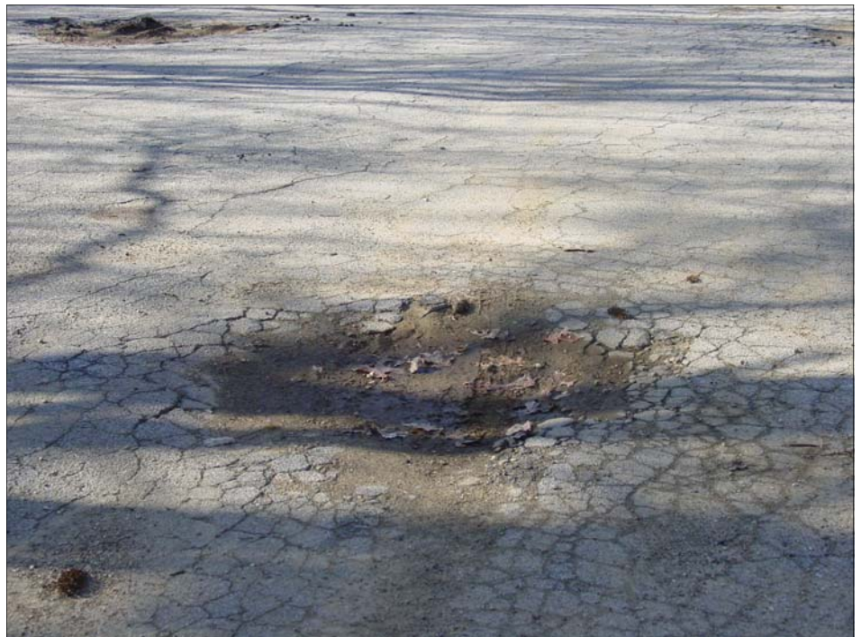
Welcome to the H.S.A - When you come through the gate into the parking lot this pot hole is there to greet you. A few years ago this hole was not there. Now it has grown to 3 feet in diameter and 6 inches in depth. Note the broken asphalt around the pot hole. In the upper left hand corner of the photo is a new area that has just failed this winter and is now starting to break up.
